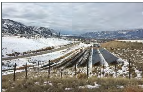
Solar array at Rifle Garfield County Airport
